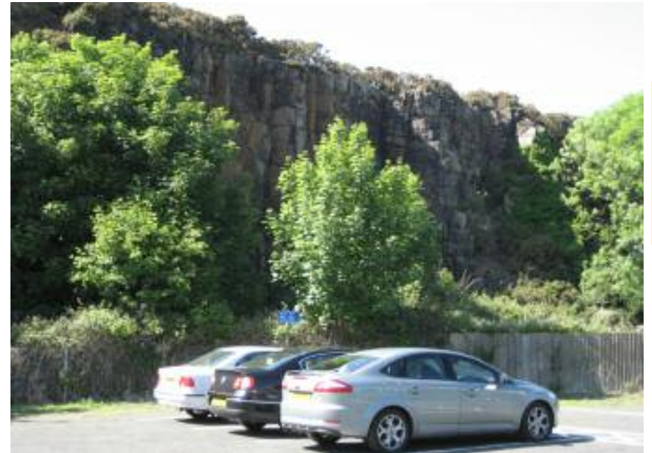
The main car park at Craster is sited within the former whinstone quarry, the faces of which are now seriously overgrown.
